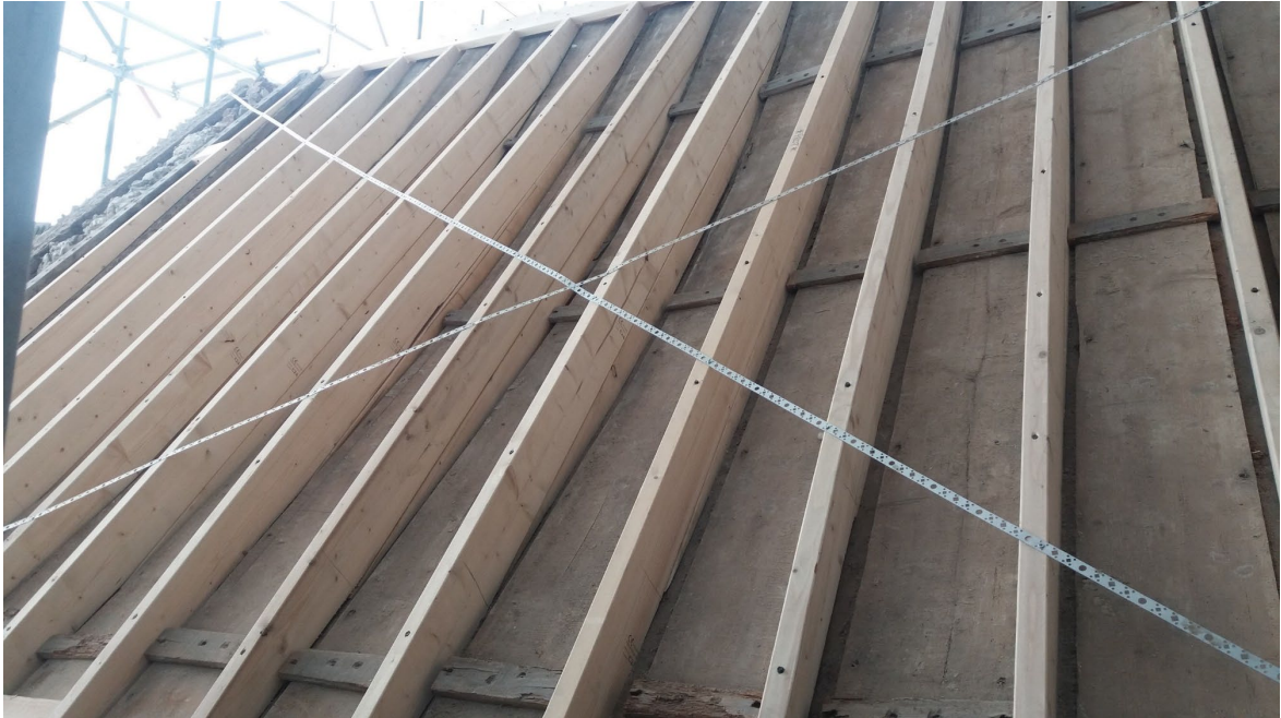
Figure 2: East end of the chancel (north slope) showing the extent of renovation and repairs preventing access to old timbers (photograph Martin Bridge)
