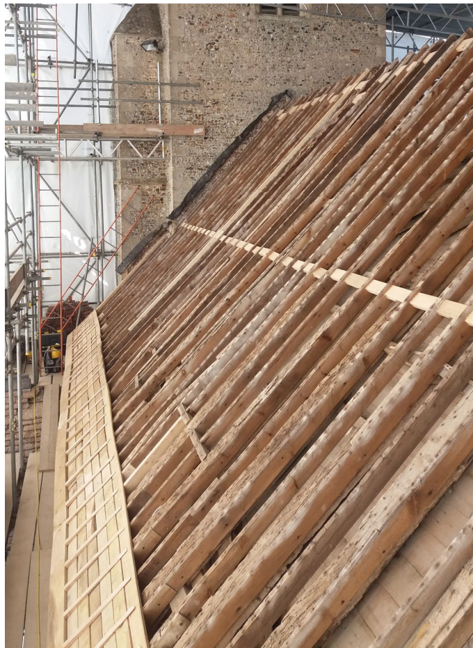
Figure 3: View of the south nave roof, looking west, showing restricted access to rafter feet and wallplates (photograph Martin Bridge)
