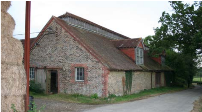
A late 19th-century covered yard building for cattle which allowed cattle to fatten more quickly and preserved the manure from dilution by rainfall. Such wide-span buildings are a feature of the western part of the Low Weald, where large estate-owned farmsteads developed on farmland reorganised in the 19th century or newly-enclosed from heath. Photo © Bob Edwards
