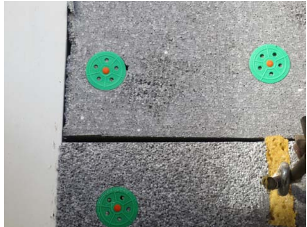
Figure 77 Poor insulation jointing
