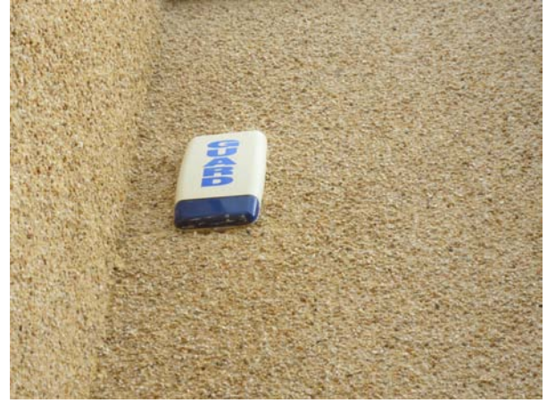
Figure 59 Alarm not removed prior to insulation
