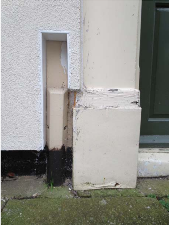
Figure 22 Gas pipe creating (required) thermal bridge
