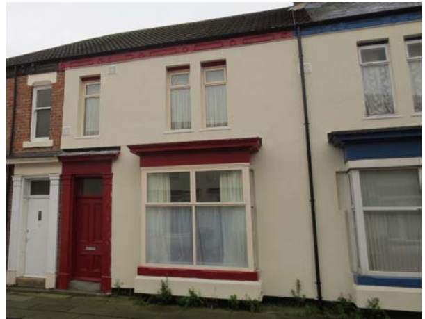
Figure 13 Untreated large window and door
