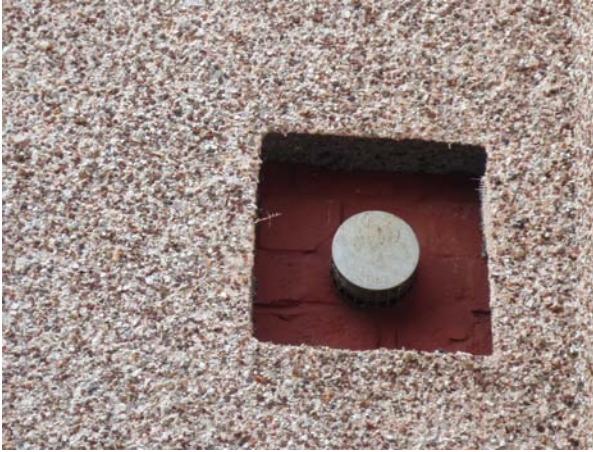
Figure 58 Unsealed insulation around flue
