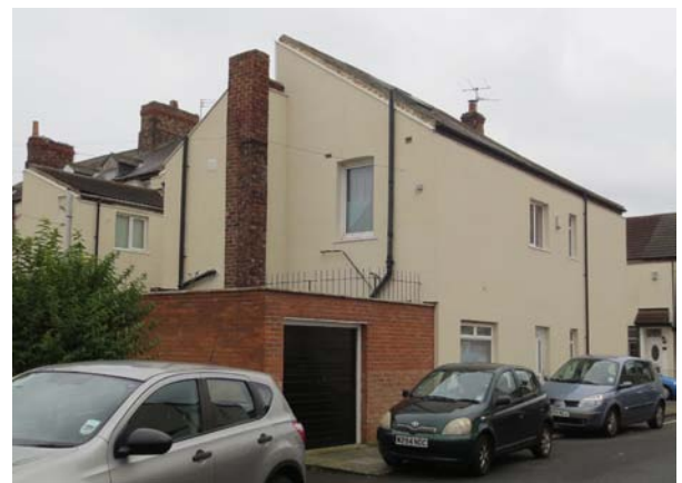
Figure 19 Note large thermal bridge
