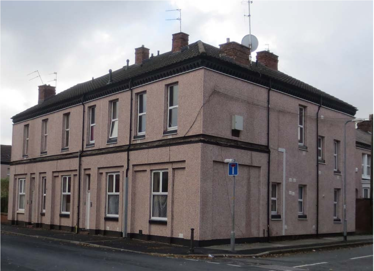
Figure 64 Note the high area of uninsulated wall area in this building; reasons for some of the untreated areas are not clear
