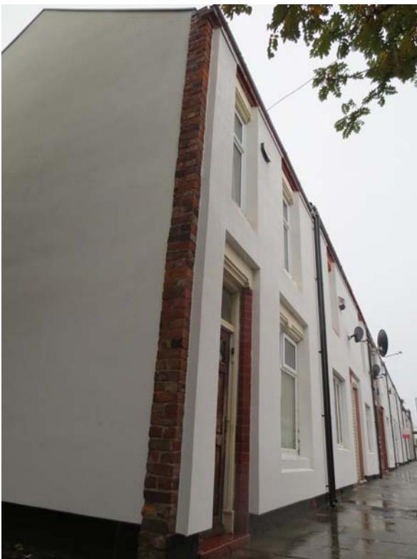
Figure 24 Note large areas of exposed building elements
