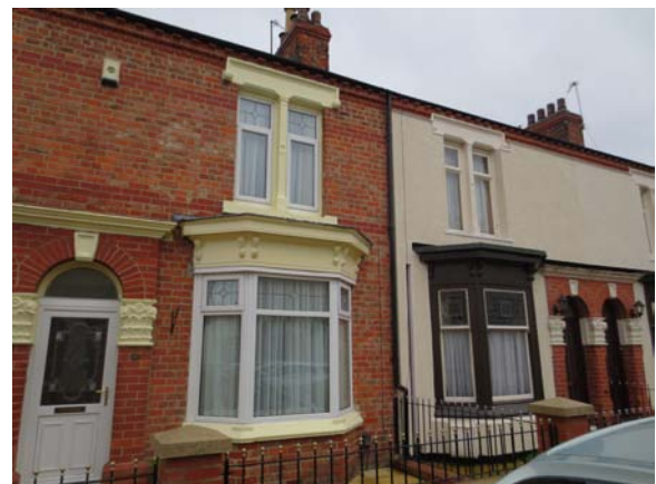
Figure 21 Large untreated areas to right-hand property
