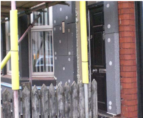
Figure 60 Burglar alarm not removed; 'squirty foam' 67
