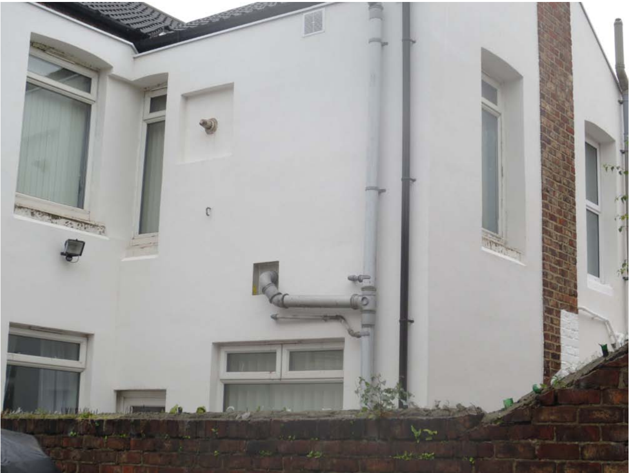
Figure 44 Note the many thermal bridges, in particular the corner bridge between the two upper windows
