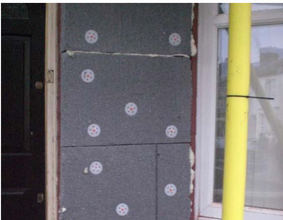
Figure 62 Poor insulation jointing 69
