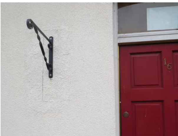
Figure 30 Note cracks in finish around plant holder
