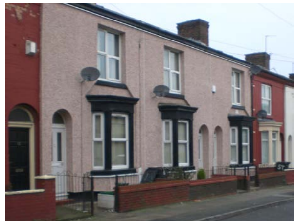
Figure 63 Note uninsulated areas above bay windows 70
