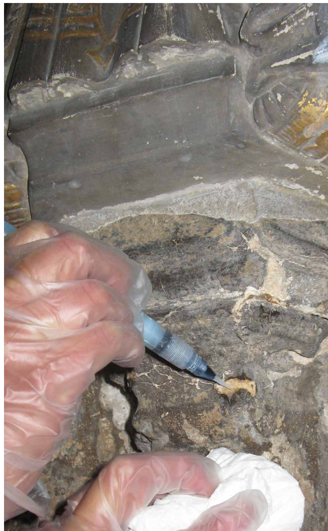
Figure 26 Norwich Cathedral. Conservator using a water brush to apply nanolime to localised decay of carved detail in the cloisters.
