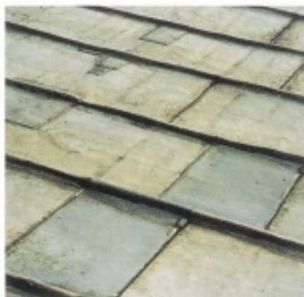
Figure 24 The large patches to the laps in the foreground suggest acid corrosion-related failures, which often first destroy the lead near the head of the lap. So do the smaller patches at the sides of the sheets, though similar damage can be caused by restrained thermal movement at tight fixing clips. The decking here is oak, probably 150–200 years old, but 35 years after re-leading, corrosion is severe.
