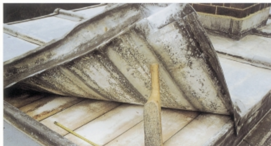
Figure 21 A typical corrosion pattern where lead has been laid directly over softwood boards in this historic house by the Thames, now used as offices. After 90 years, the underside of the lead is still in relatively good condition, but moisture and acids have caused some corrosion over the boards, while areas above the gaps are passivated. Note the heavier corrosion under the nosing, where trapped moisture is less readily able to disperse.
