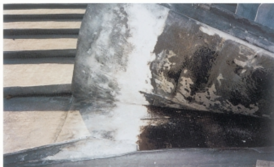
Figure 22 At this church in Yorkshire, roofing felt was used to protect the lead from acid vapours from the oak ceiling/decking. Although much of the lead has been protected, local membrane failure together with some water ingress has led to localised corrosion which in places has perforated the lead sheet.
