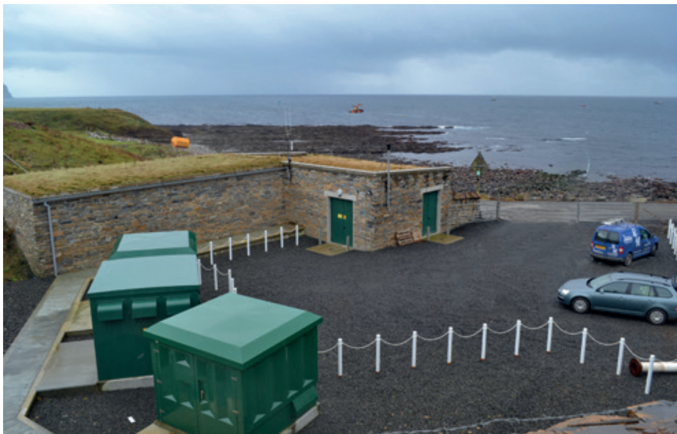
Onshore facilities at the EMEC test site at Billia Croo, Orkney, with the test site itself in the background. Image © Antony Firth/Fjorðr.
