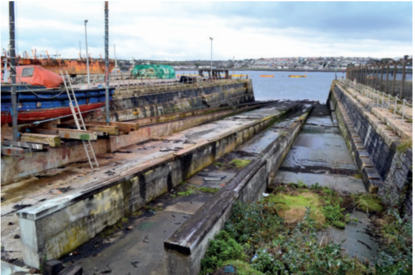
Historic structures such as this slipway at Pembroke Dock – which was second only to Plymouth for building Royal Navy ships in the mid-late C19th – may be capable of sensitive reuse in supporting the wave and tidal energy sector. Image © Antony Firth/Fjorðr.
