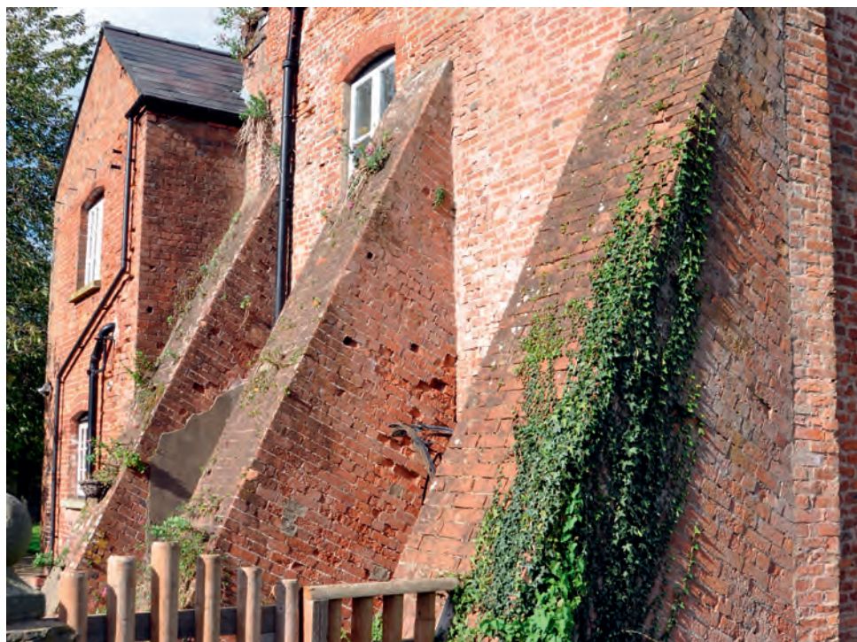
Heavy 19th-century brick buttresses intended to provide a counter-thrust to a flank wall. If buttress foundations are not well designed or constructed, settlement can occur which can pull the wall further out of plumb, rather than restrain it.
