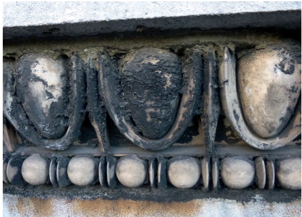
A heavy crust of calcium sulphate has developed over centuries: this element of the building has not been cleaned since it was built in 1821.
