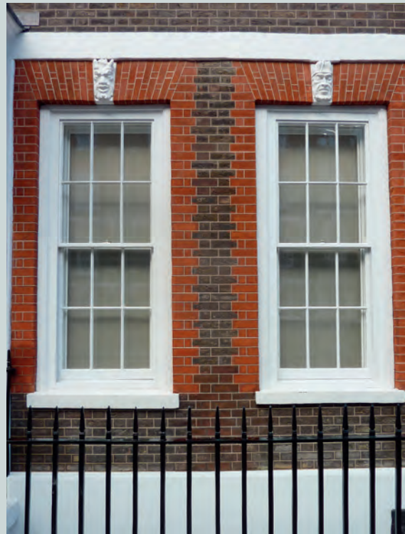
Restored tuck pointing on the façade of an early 18th-century town house in Westminster, London.
