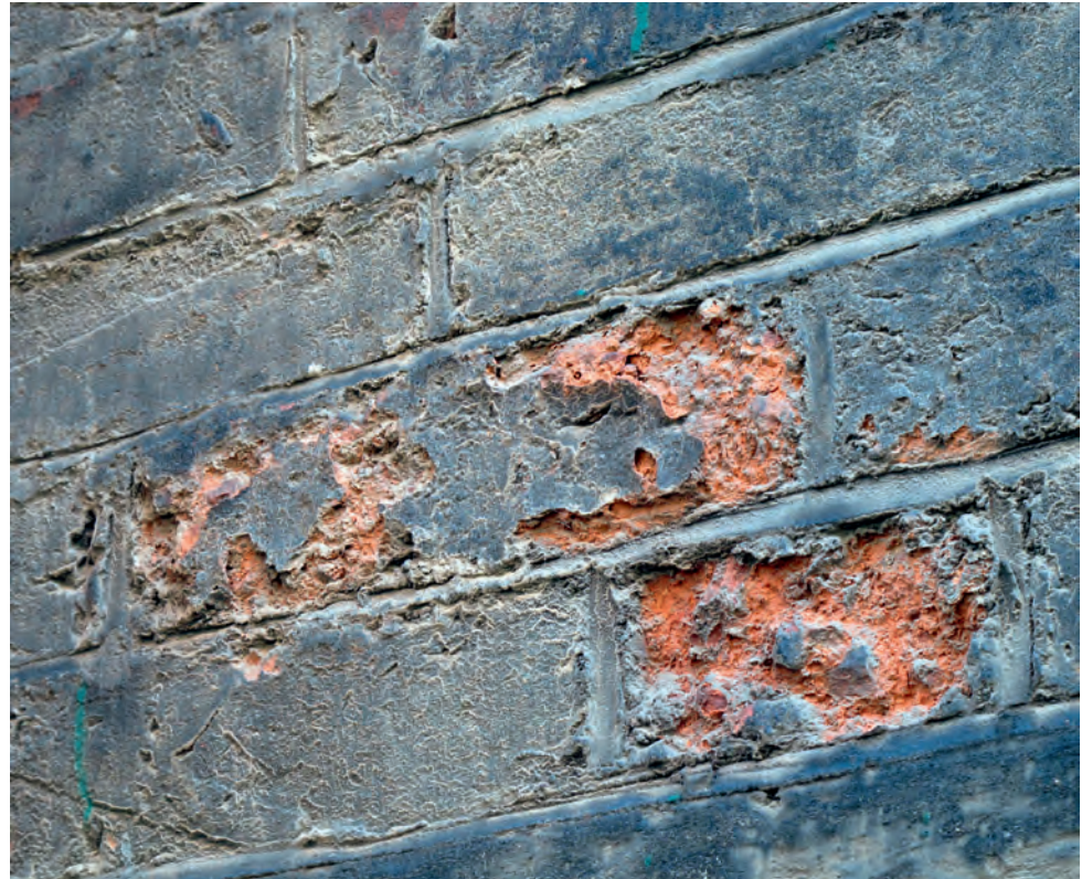
Accumulated salts and soiling can form a skin on the surface of bricks which may blister and become detached due to differential moisture and thermal movements, and salts.
