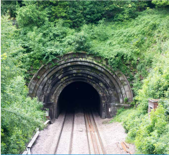
Milford Tunnel North Portal, Derbyshire, upgraded to grade II* for its unusual design of concentric rings.
