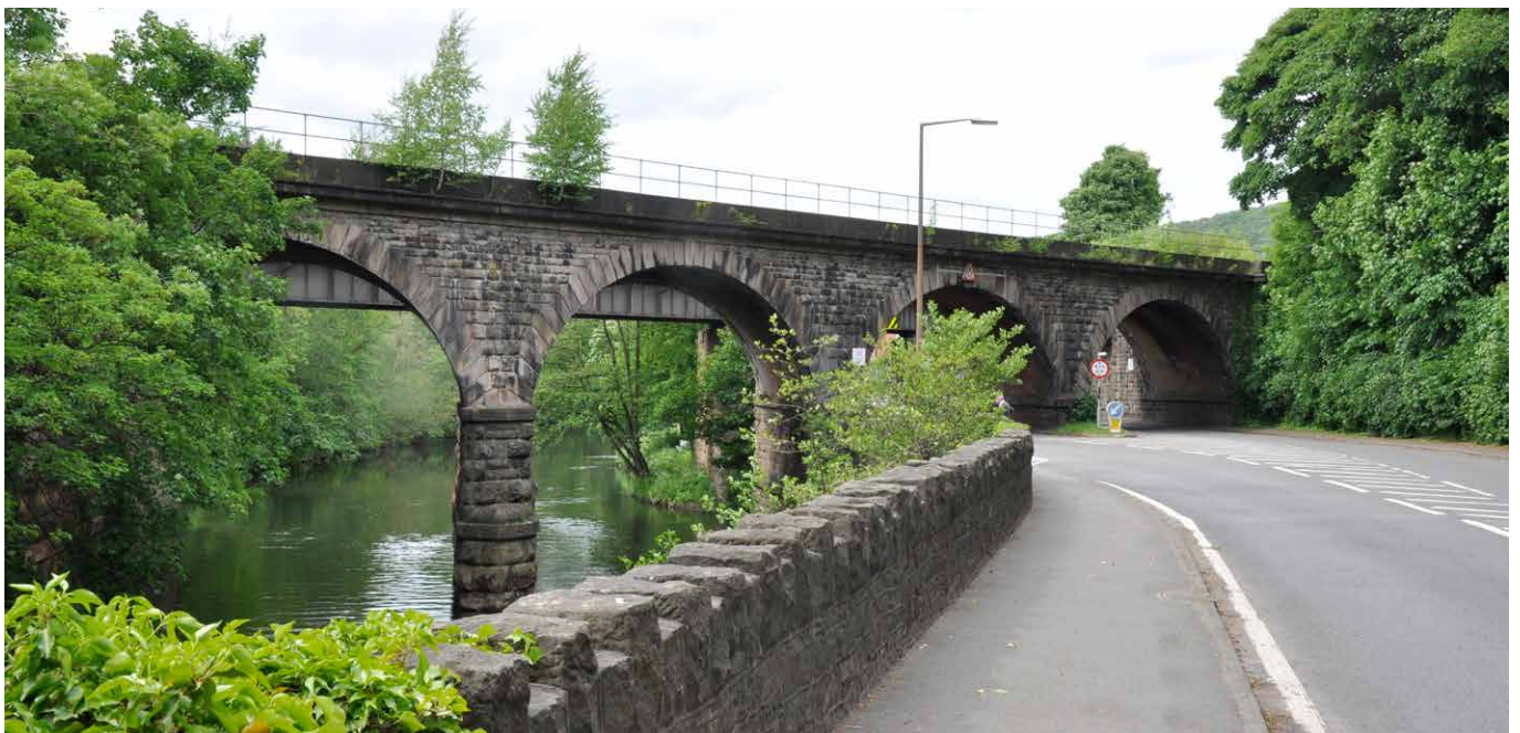
The fine skew arches of Derwent Viaduct, Derbyshire, listed at grade II* during the designation review. © Alan Baxter and Associates
