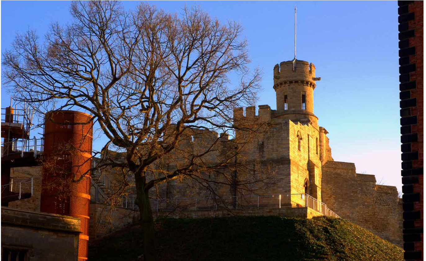
In order to create the full circuit wall walk and enable people with limited mobility to enjoy spectacular views over Lincoln, the Castle, The Cathedral and surrounding area a new stair and lift tower was created, replacing haphazard concrete access points around the Wall. It responded to its visually sensitive location by limiting height and the corten steel outer coating is consciously different whilst maintain an austere aesthetic in keeping with the prison and Castle. © Andrew Tryner, Lincolnshire County Council
