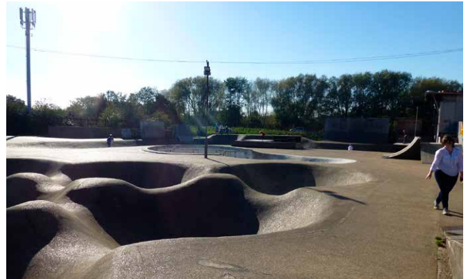
The Rom skatepark, Havering, built in 1978 to designs of Adrian Rold of G-force. The grade II listing is focused on the shotcrete surface with its bowls and hollows, and not the temporary ramps and clubhouse. © Historic England
