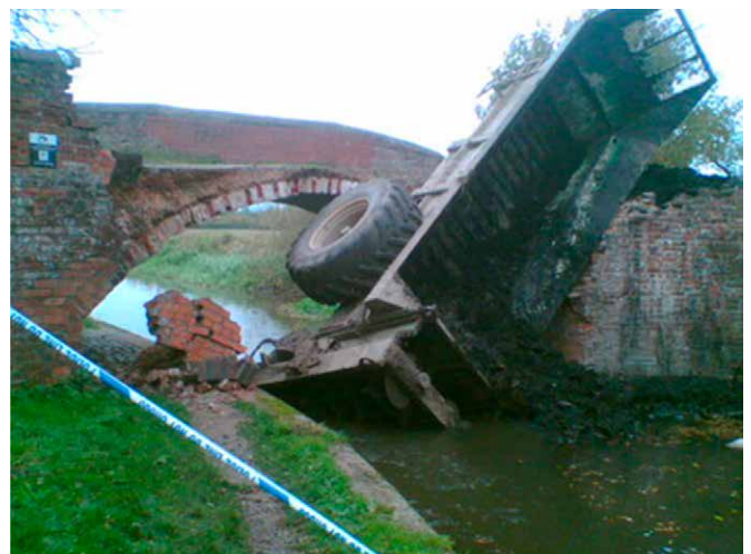
Vehicle damage to bridges is not uncommon and repairs could be covered by the national LBCO. © Canal & River Trust
