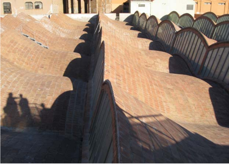
A Spanish Anchor Point: the roof of a modernista textile factory, Terrassa, now the Catalan Museum of Science & Technology.
