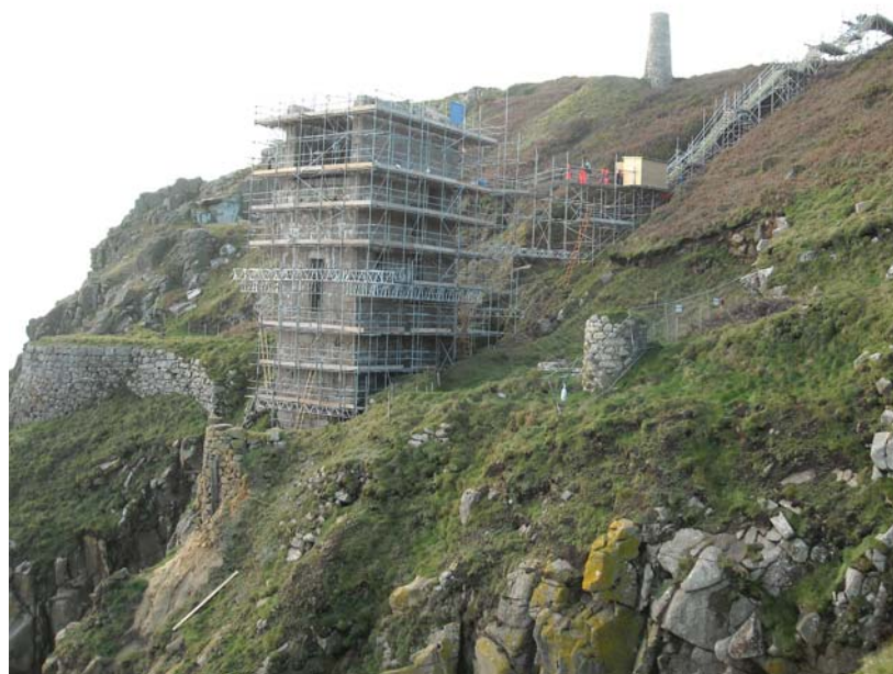
A view of the scaffolding and access stairway on the Engine House on Old Engine Shaft during consolidation work at Trewavas in West Cornwall.
