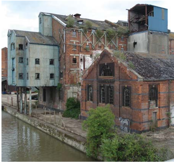
Provender Mill, Baker's Quay, Gloucester. This 19th-century grain warehouse is designated as a listed building and on the City Council's Buildings at Risk Register.
