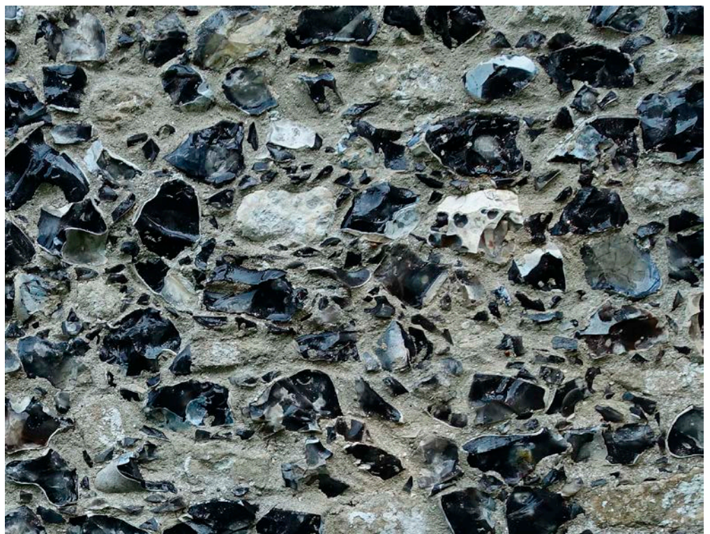
Figure 25: Church of St Mary, Santon Downham. Knapped Quarry Flint with Totternhoe Stone blocks.
