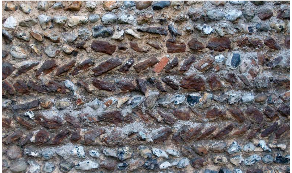
Figure 36: Church of St Mary of the Assumption, Ufford. Red Crag ironstone and Quaternary Flint nodules.
