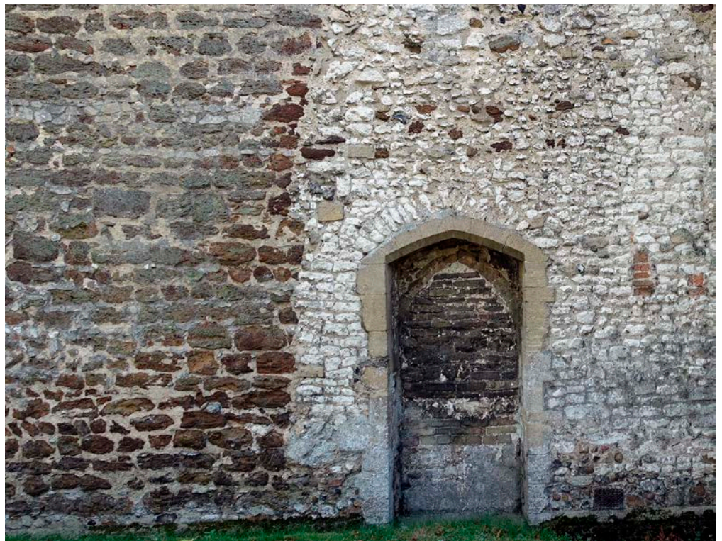
Figure 23: St Mary's Church, Lakenheath. Roughly coursed chalk and more regularly coursed carstone, with Lincolnshire Limestone dressings.
