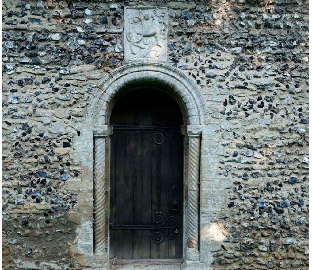
Figure 24: Church of St Mary, Santon Downham. Quaternary Flint walls with a Totternhoe Stone arch and Barnack Stone dressings.
