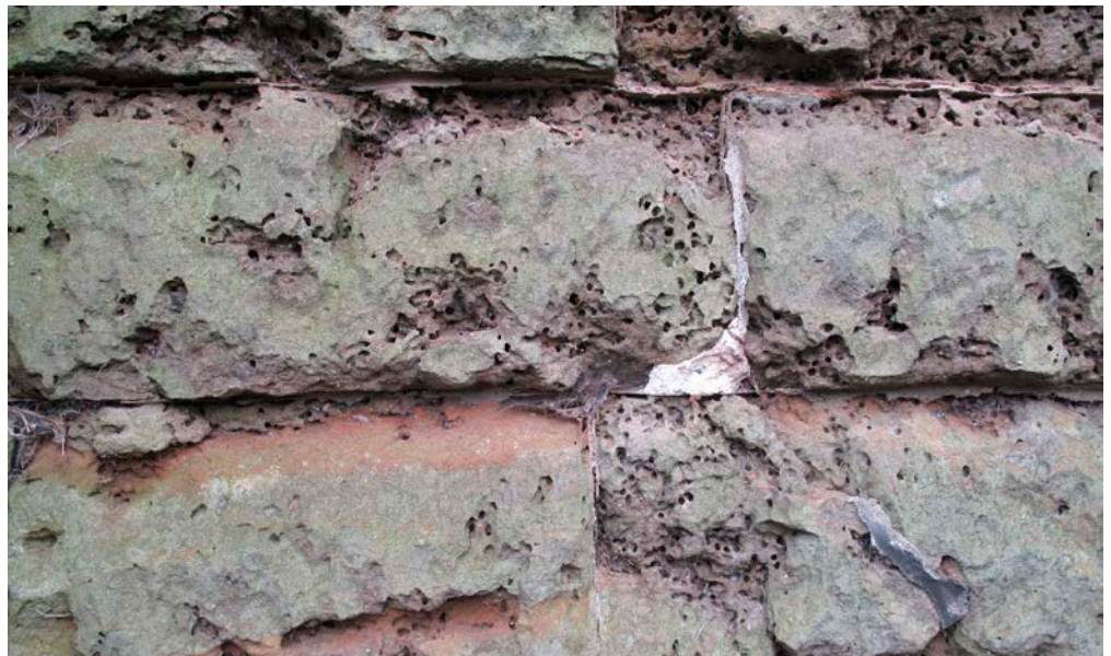
Figure 14: St Mary's Church, Tetford. Spilsby Sandstone.
