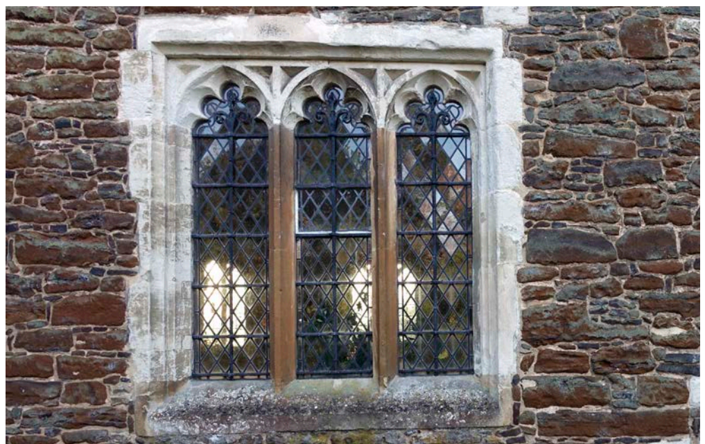
Figure 34: Church of St Mary, Great Brickhill. Totternhoe Stone windows with Bath Stone repairs.
