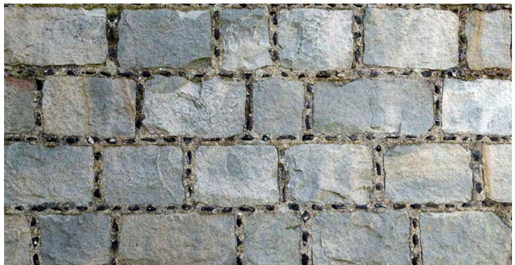
Figure 49: Detail of the walls of the Church of St Michael and All Angels, Halton. Sarsen stone blocks with flint galleting.
