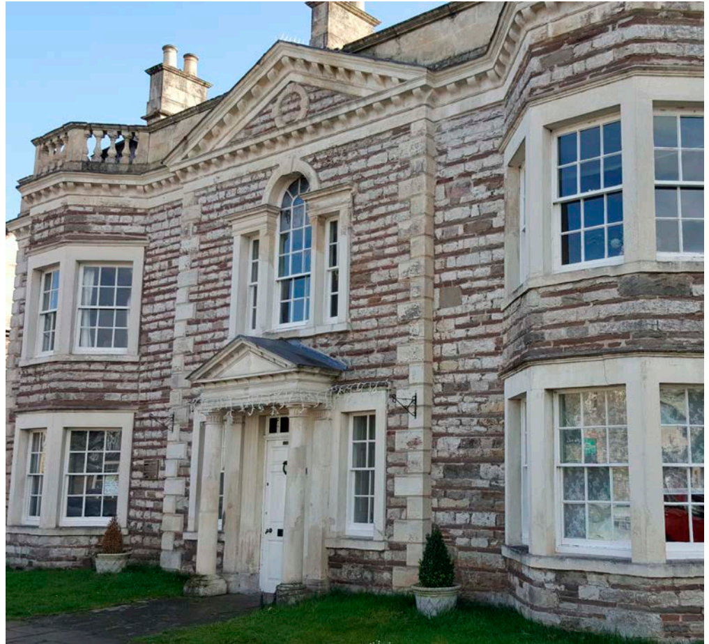
Figure 9: 64 Rounceval Street, Chipping Sodbury. Thin, dark bands of Cromhall Sandstone alternate with thicker courses of pale grey Lower Carboniferous Limestone.
