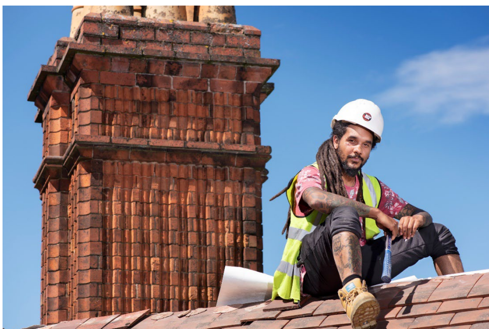
A builder sits on the roof of Highbury Hall in Birmingham during a restoration project. © Historic England Archive
