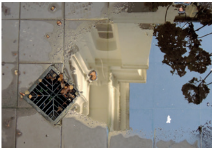
Water will not run uphill into a drain, and yet poorly-positioned drains are common.
