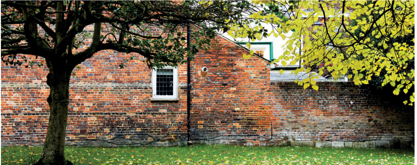
'Rising damp' is an excellent example of how many different sources of moisture can produce very similar symptoms. At the right, this wall shows the classic symptoms often attributed to capillary rise from groundwater: a zone of salt damage and staining, separating a dry area above from a wet area below. Closer examination shows that the majority of the wall is fine – which it would not be if groundwater were the issue – and that the source is in fact run-off from a glass roof behind, saturating the wall and percolating downwards. Other common causes of this damage pattern include splash-back and plumbing leaks.
