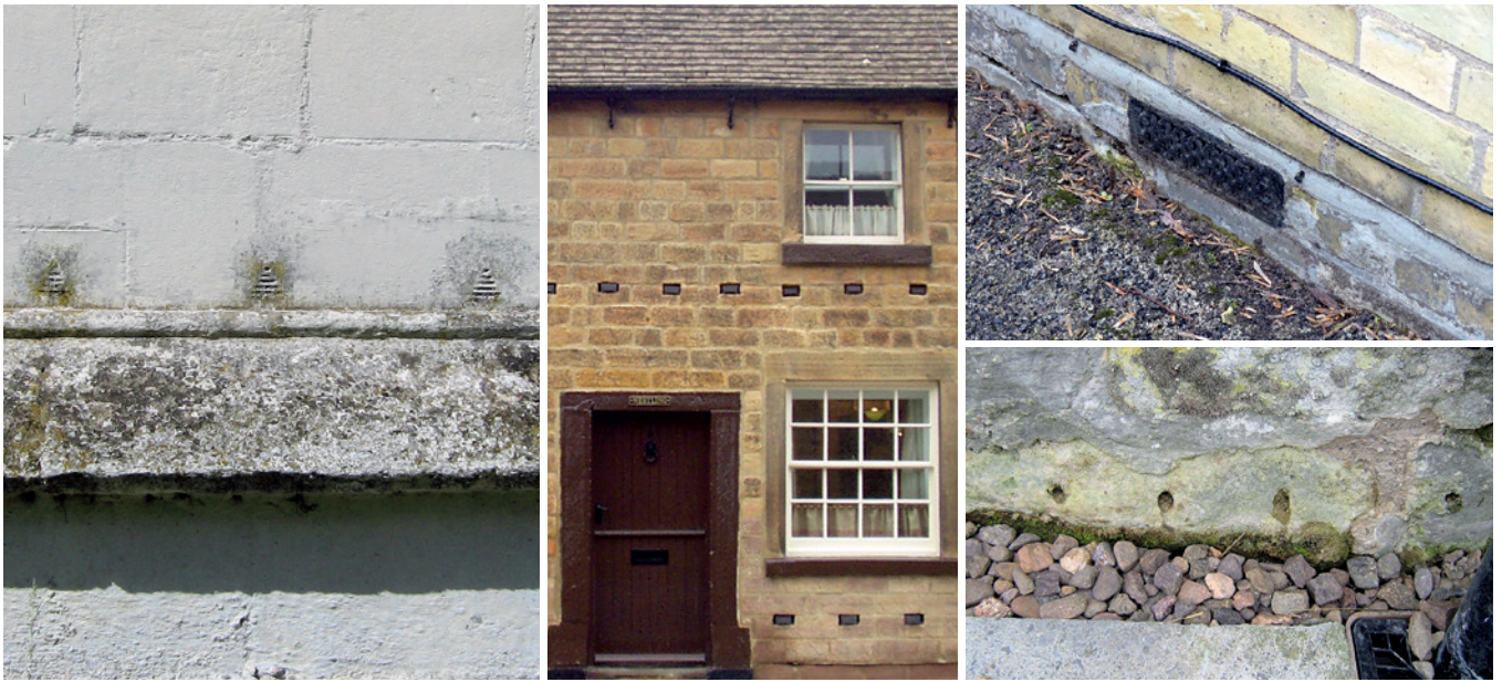
Failed remedial treatments are often based on wrong notions about the behaviour of water. The operation of Knapen tubes, for example, is based on the idea that humid air is heavy and so will fall. In reality, humid air rises.
