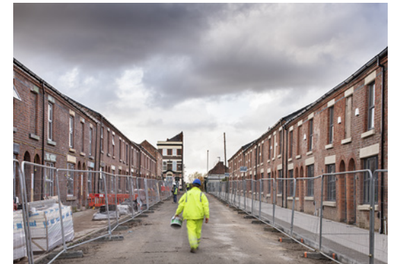
Converting Victorian terraces in The Welsh Streets, Liverpool. Retrofitting heritage properties has a significantly lower carbon impact than building anew.
